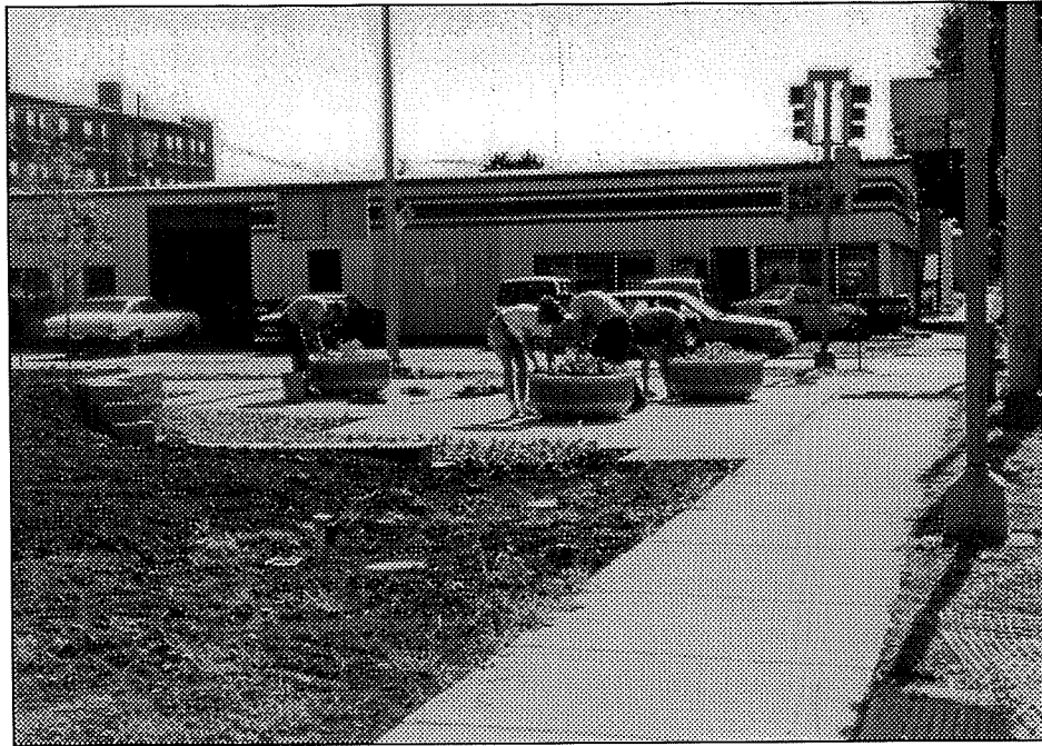
Mini park construction at the corner of Wright St. and University Ave.
