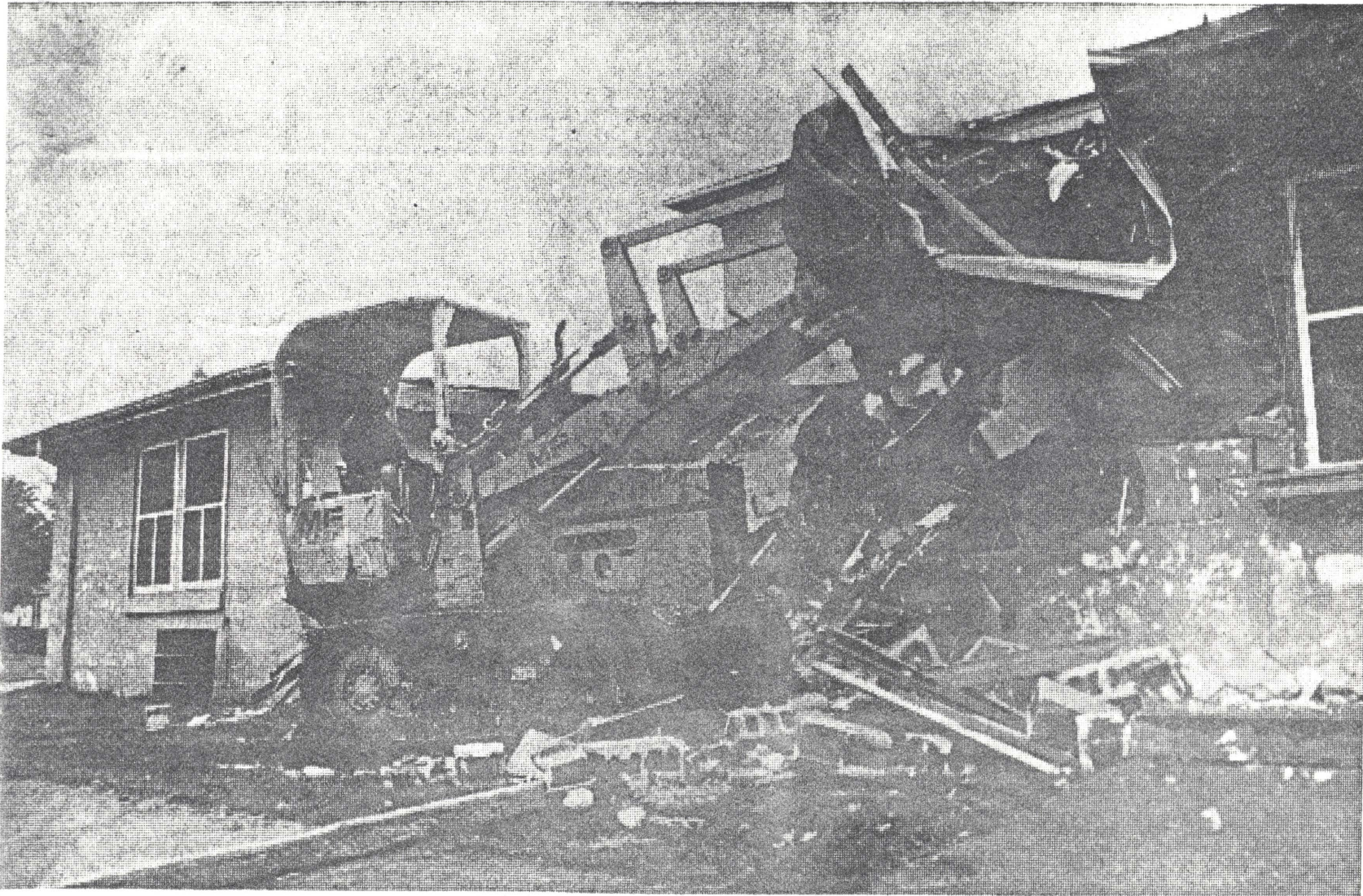
Months to build, years to serve northeast Champaign—Douglass Center comes down in minutes this morning
