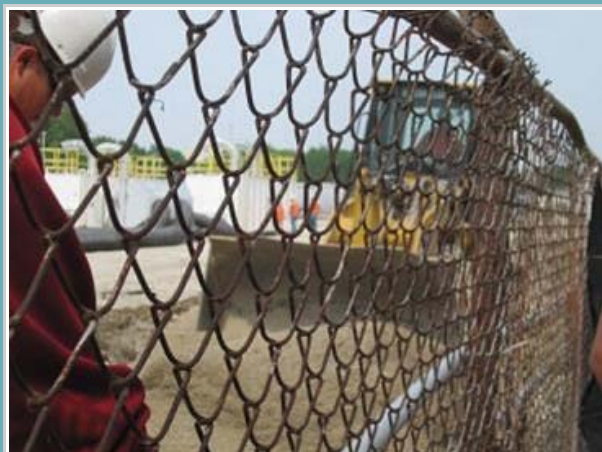
Picture by: Sean Powers/Illinois Public Media/A bulldozer removes soil that is suspected of having traces of the pollutant coal tar on the corner of 5th and Hill Streets in Champaign on Thursday, June 9, 2011.
