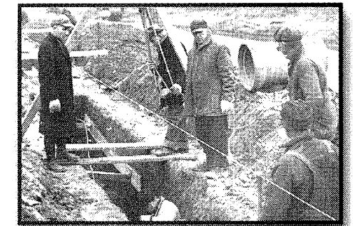
WPA storm drain improvement at Prospect & Vine Photo courtesy of Champaign Country Historical Archive, The Urbana Free Library, Urbana, Illinois
