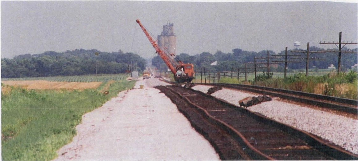
To handle the great increase in traffic on the NS line, the railroad built new passing sidings, and here one under construction near Sadorus is seen in June 1998.
