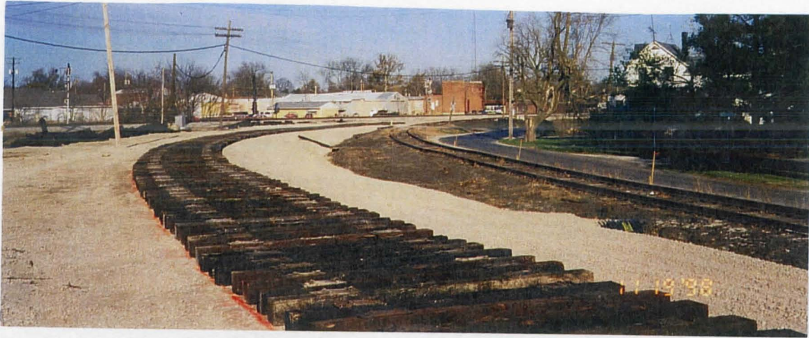
Ties for the new curve line being built at Tolono to join the NS and IC lines, as seen on in 1998.
