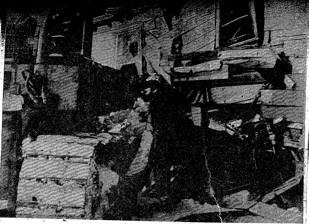
News-Gazette Photo by Joe McNamara 'DOZER BLADE TAKES FIRST URBAN RENEWAL BITE ... and the walls came tumbling down in 15 minutes
