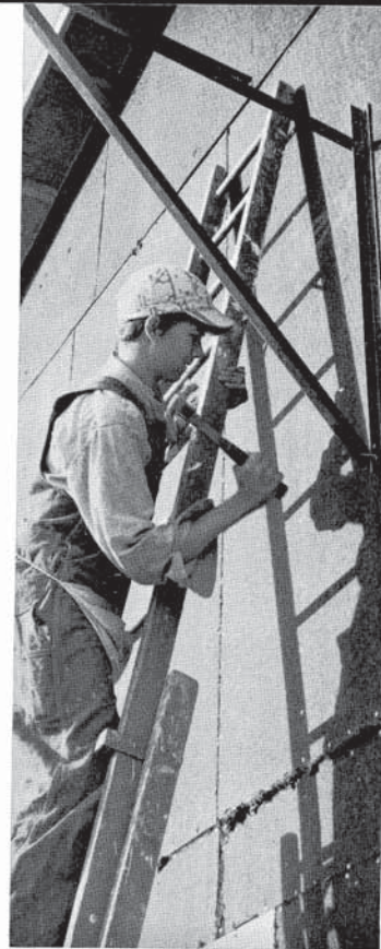
Tom Edmison hammers on the exterior of the house while good weather prevails.
