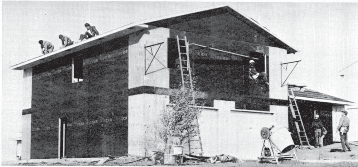
Building Trades students work on the project house one fall morning under the watchful eye of Mr. Robert Pittman.
