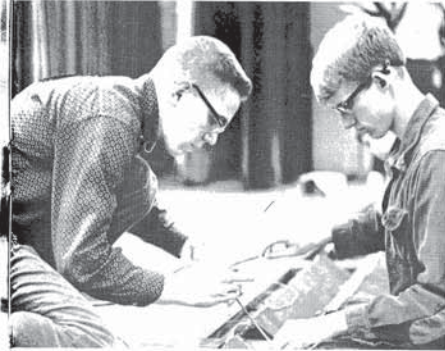
Mike Fredericks and Alan Brown display technical knowledge in wiring the lights.
