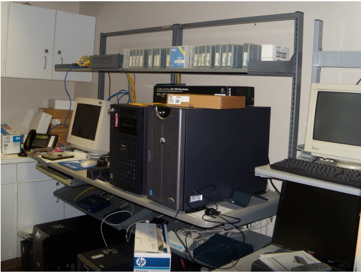
Server room located in the administrative building.
