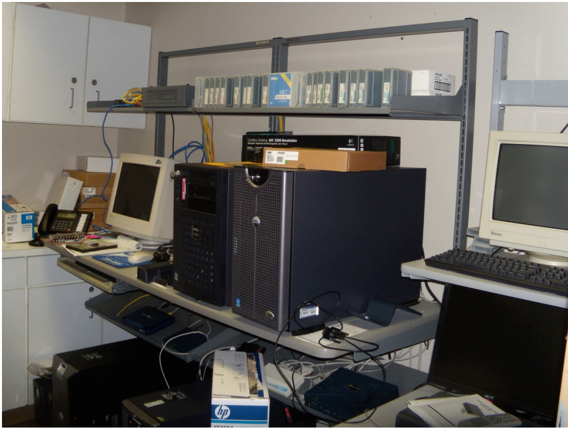
Server room located in the administrative building.
